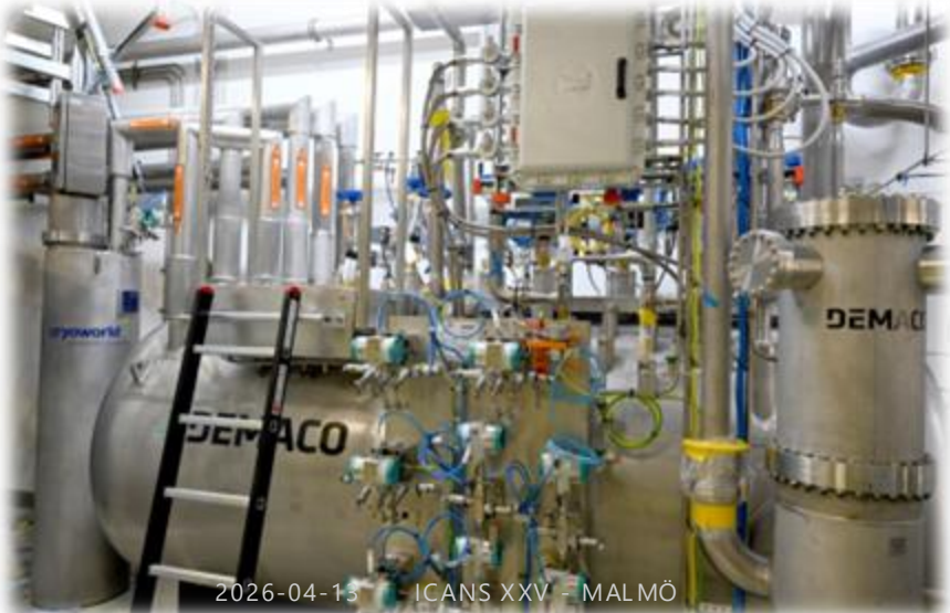
Cryogenic Moderator System Junction Box
