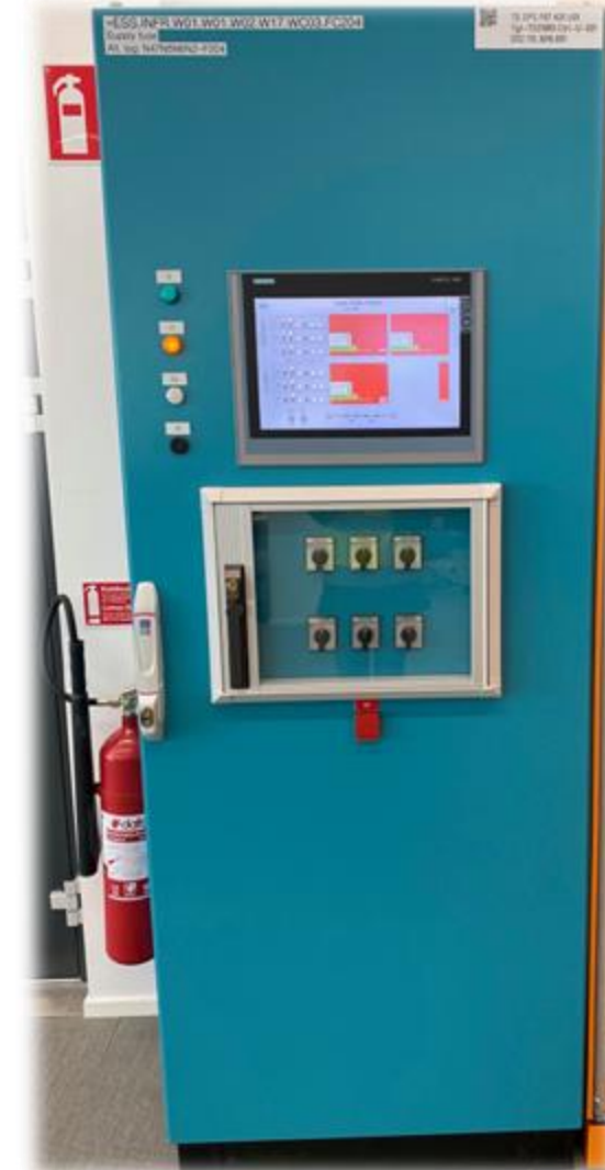
TSS control room cabinet
