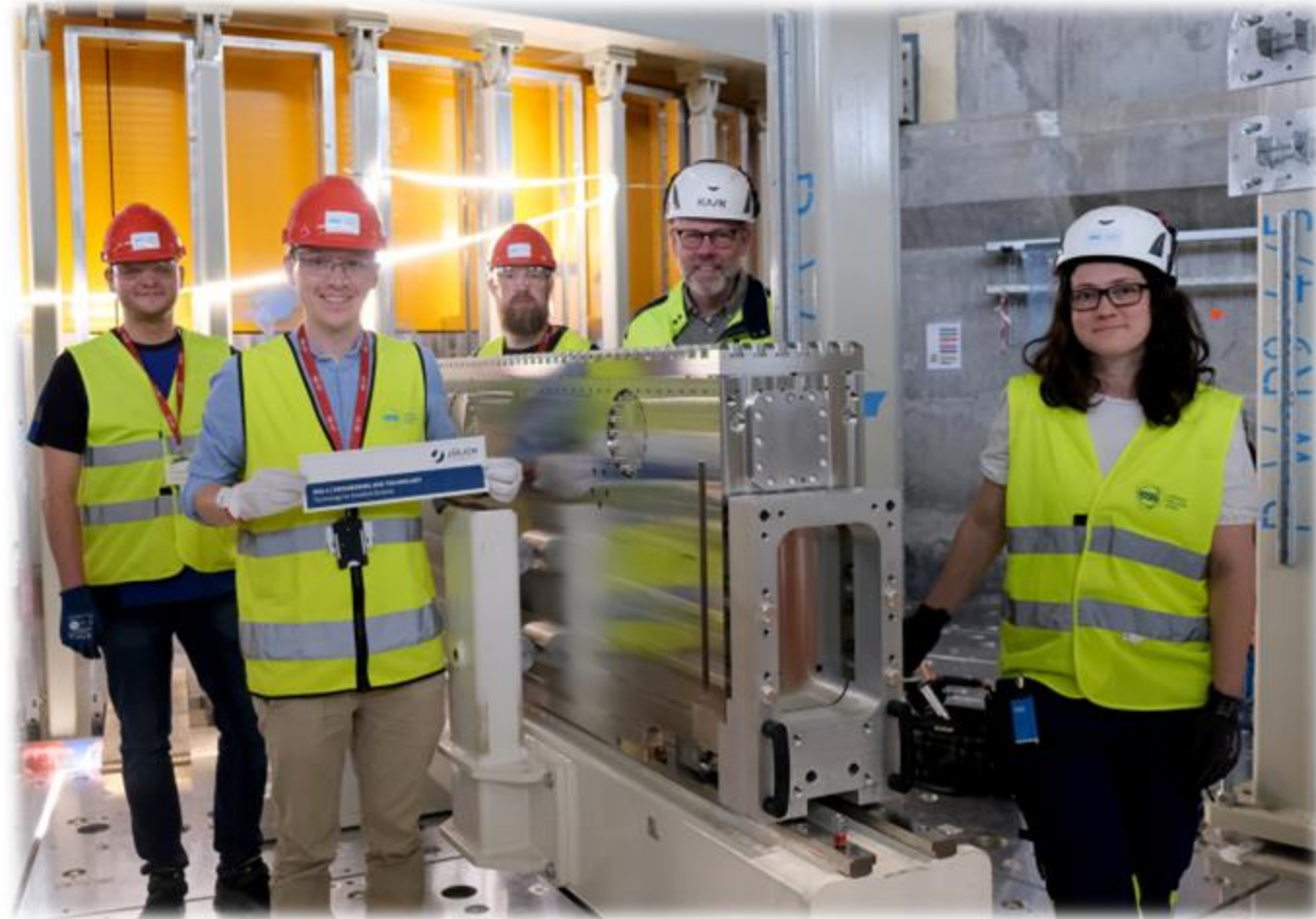
Last Neutron Beam Port Insert being installed together with in-kind partner FZJ
