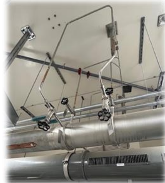
TSS venturi tube flow measurement
