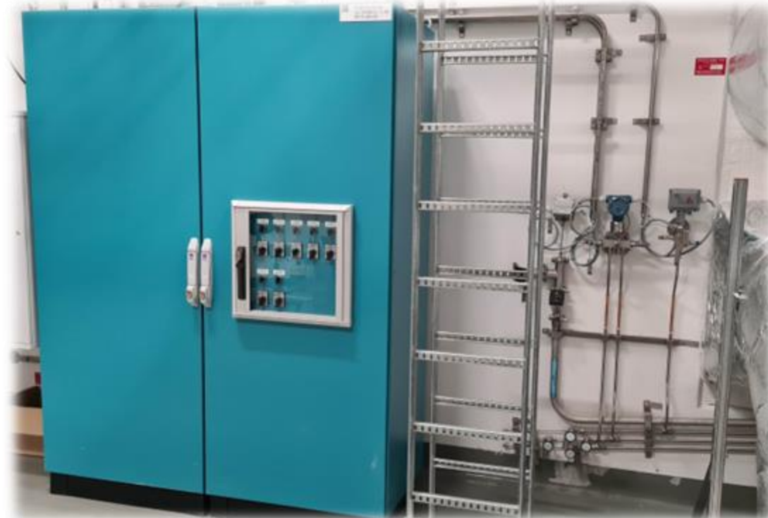
TSS field control cabinet
