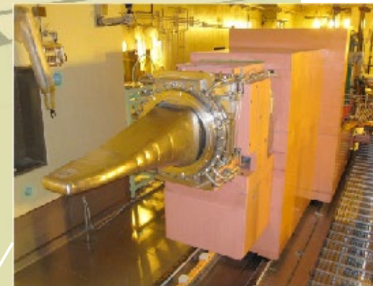
Maintenance area (Hot cell)
